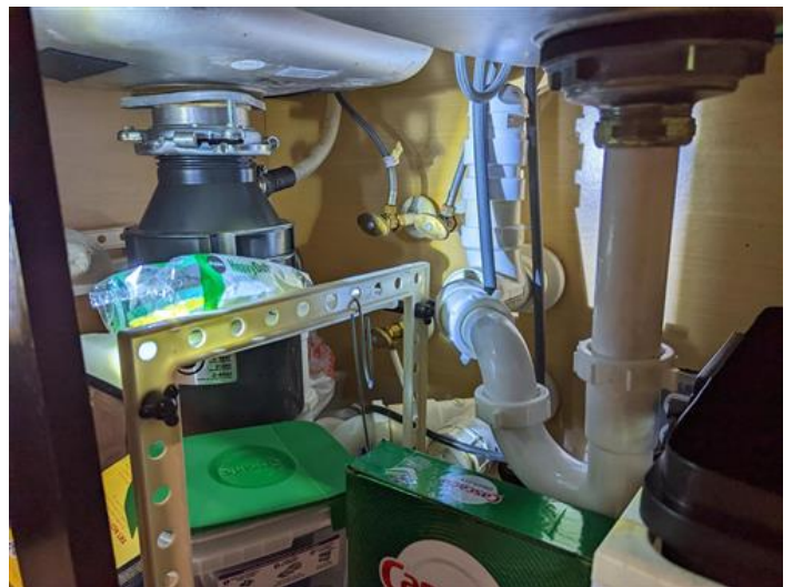
Kitchen Sink Plumbing
