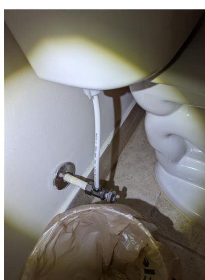
Toilet Sink Plumbing
