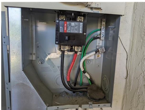
Main Panel Wiring
