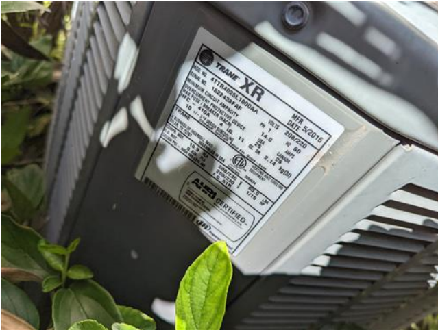
HVAC Condenser Label
