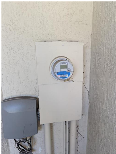
Main Electrical panel and meter
